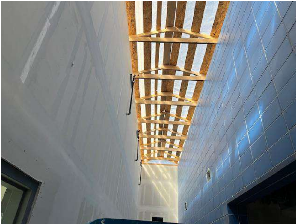
Fire Suppression in Skylight Well
