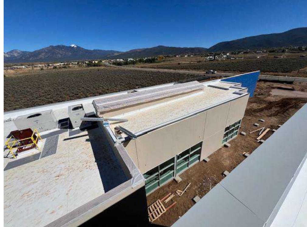
RTUs and Walk Pads / Parapet Caps
