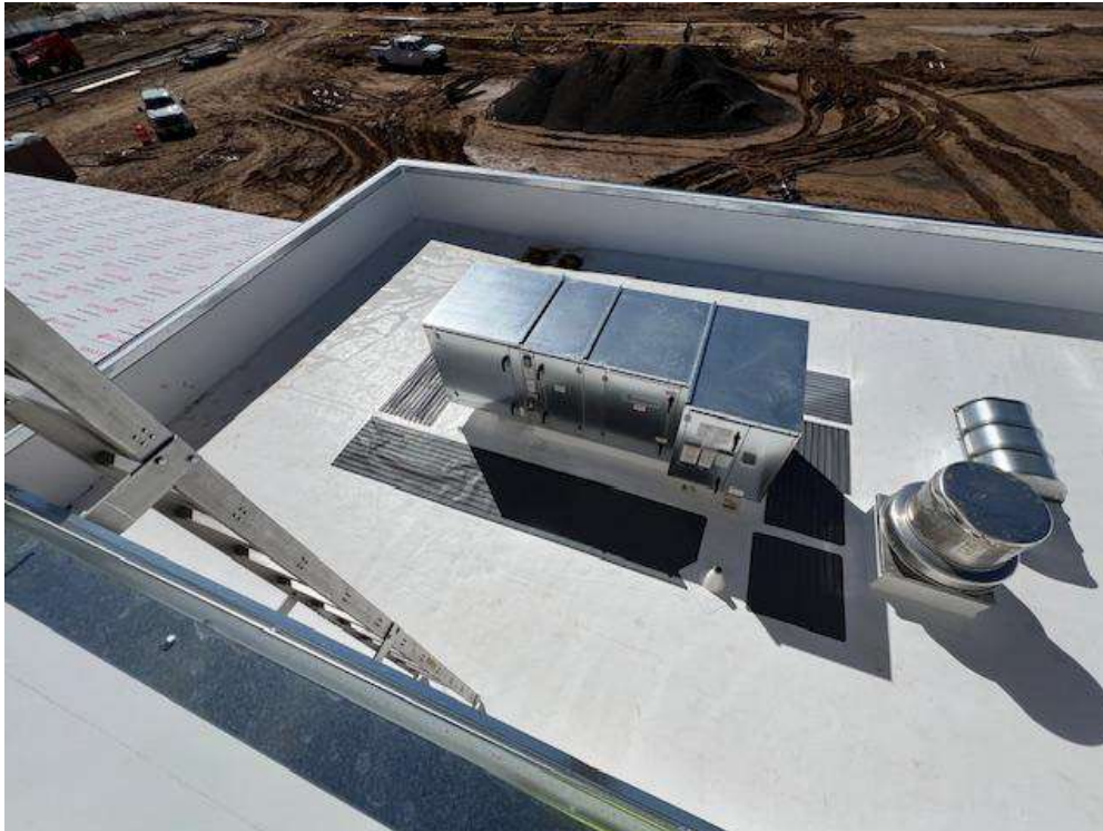
RTU and Walk Pads / Exterior Access Ladder
