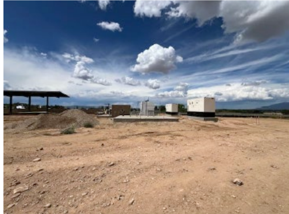
Generators and Fuel Island Canopy
