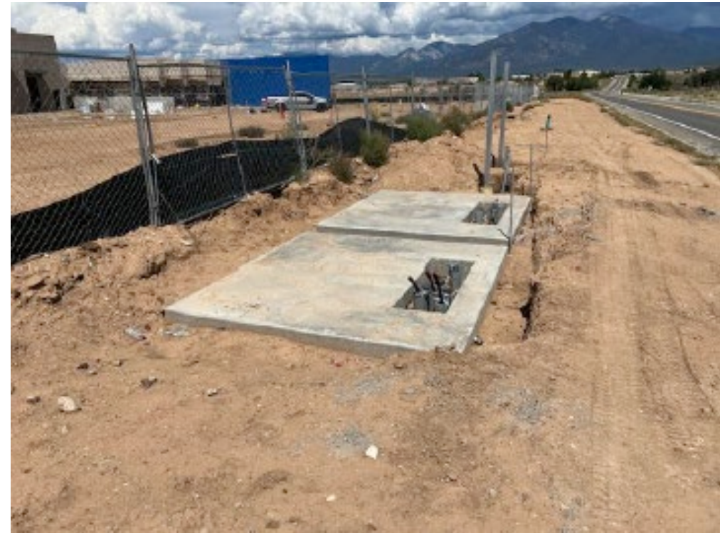
Transformer Pads Along Salazar
