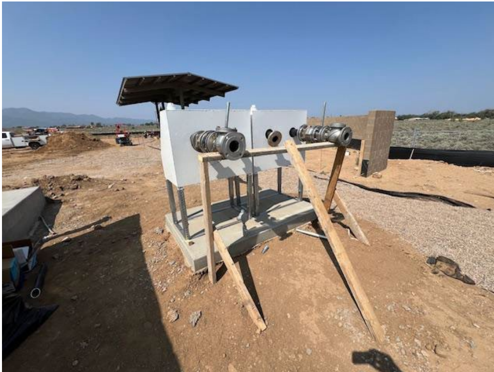
Fuel line equipment
