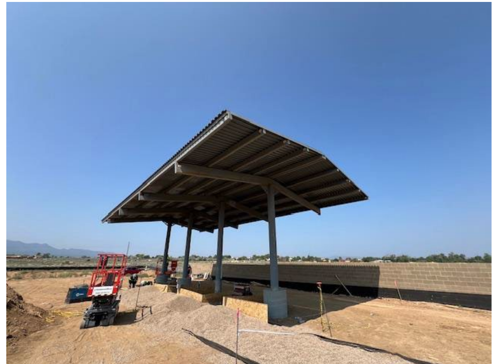
Fuel island and canopy
