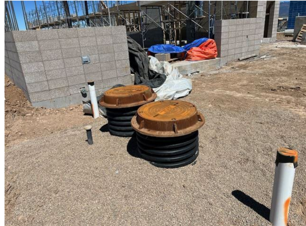
Oil water separator
